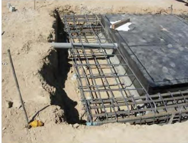
Picture 8 - Conduit Connection
